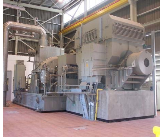
PRG Granary 9.24 MW Cogeneration Plant Thailand
