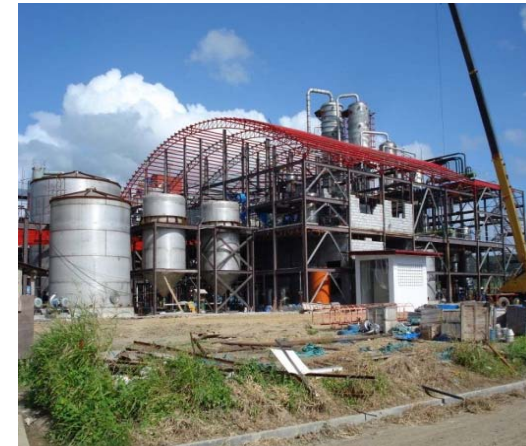
San Carlos Bioenergy Ethanol Plant Philippines
